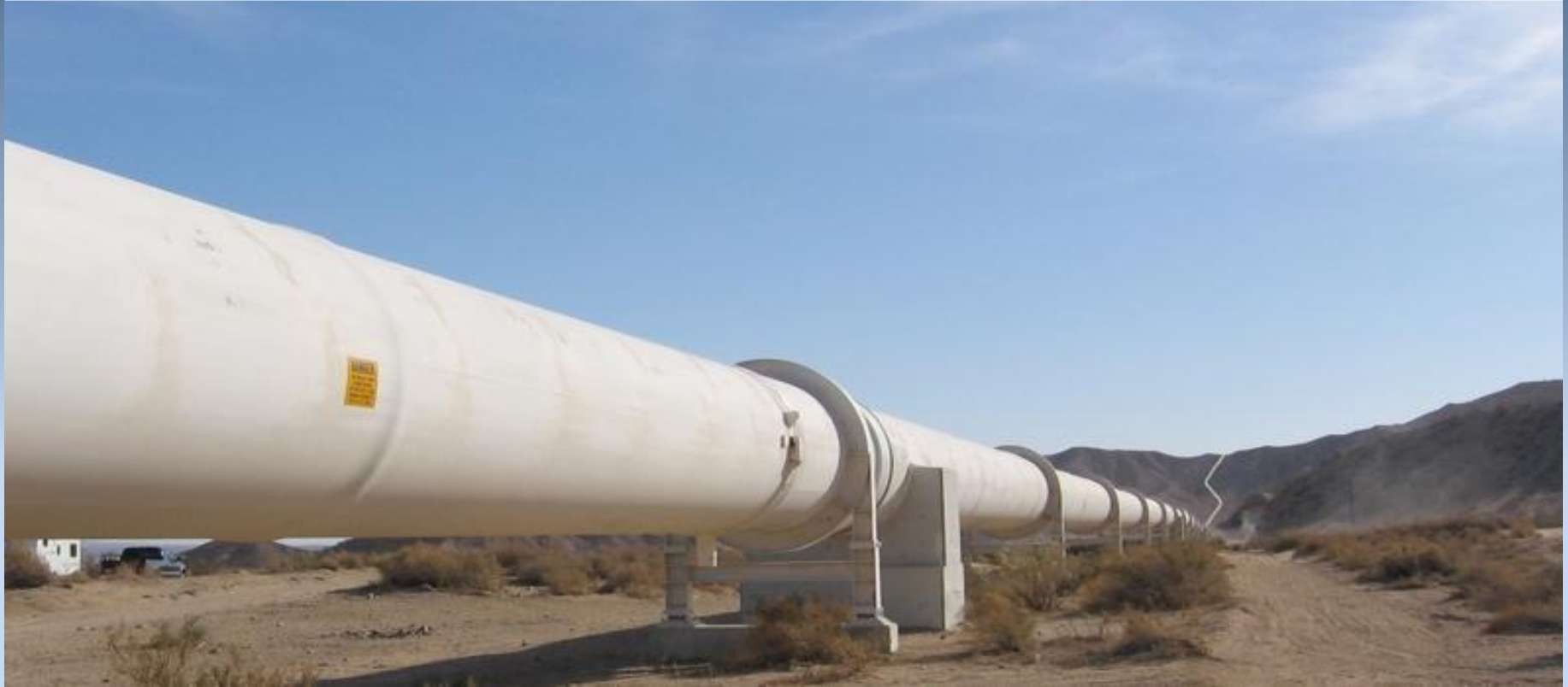
Water Transmission Pipeline
